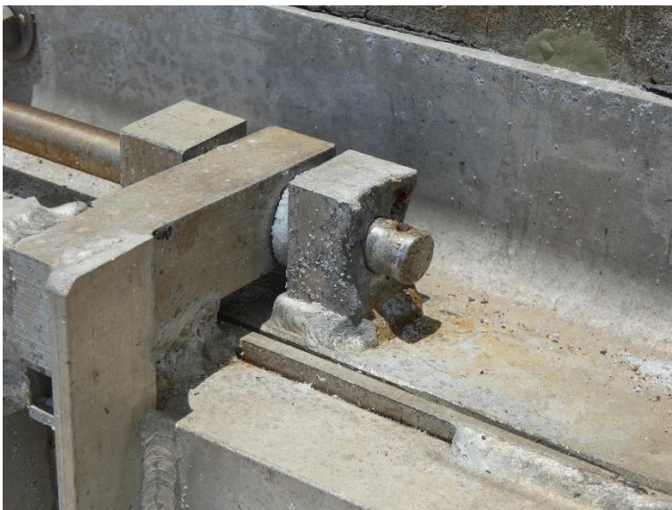
Photo of northern cotter pin which has corroded away.
